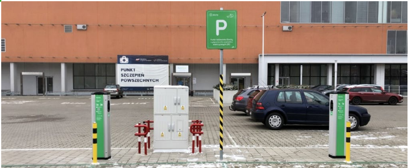
Electric vehicle charging stations on campus B. Source www.elo.city
